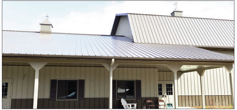
The exterior of the education center is nearly done, but much work remains inside.
