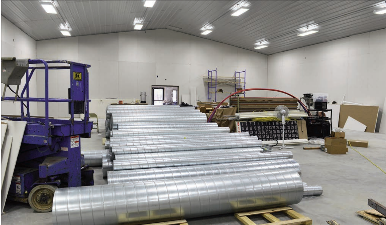
Air ventilation pipes wait to be installed in the large room of the new education center. The pipes cannot be hung until the taping and painting is done. Volunteers are needed to tape, sand and paint the interior of the building. When sessions at Legionville Camp, on North Long Lake near Brainerd, begin in June, the large room will not be in use. Classrooms in the building, however, will be used.
