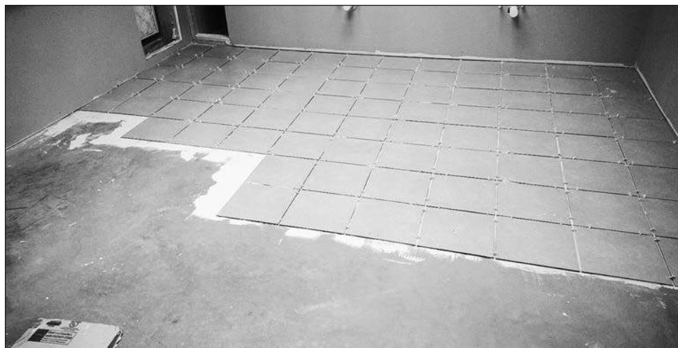
LEGIONVILLE WORK -- The painting is done and much of the finishing work is being completed at the education center at Legionville School Patrol Camp near Brainerd. The camp will open, using the new education building, on June 14. A grand opening event is scheduled for the Camporee this September.
