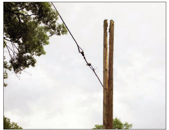
A stabilizing line from a utility pole sheared another pole right down the middle during the storm.
