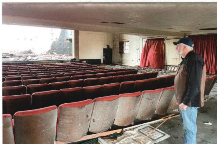
American Legion Post 26 Commander Wendell Gugu surveys the extensive damage to the movie theater located inside the post home in Mayfield, Ky. Photo by Henry Howard
