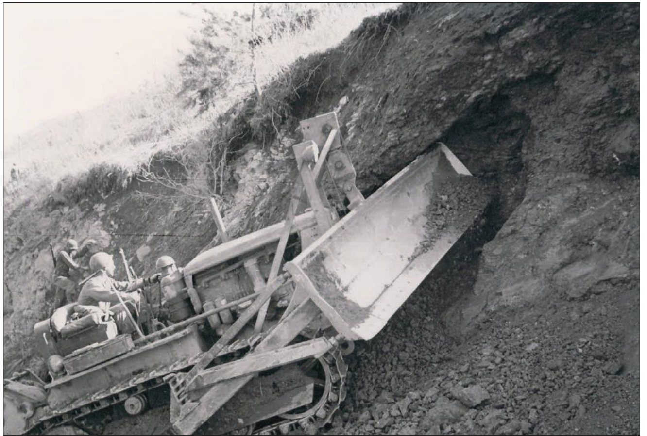
The dozers often had to cut into river banks to carve out a road in Korea. The right track sometimes was on the very edge of the road, and sometimes it was over the edge. Schulte says he tipped the bulldozer over four or five times in Korean, once in the water with the dozer on top of him. To his left are the two rifles he always carried with him while working.
